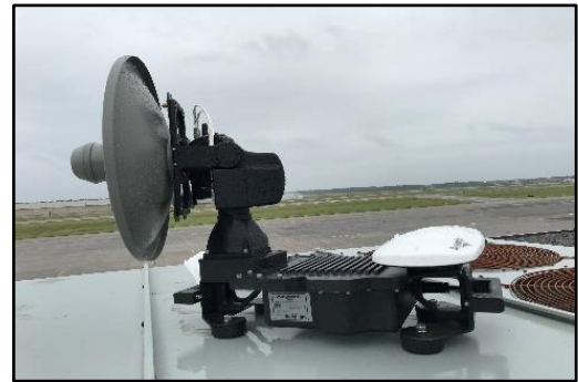
MTS deployed post-Hurricane
